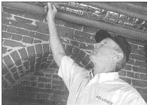
Brian Kelleher of Kelleher Corporation inspects the Unico System supply tubing used in the installation at the historic Brandon Plantation.
