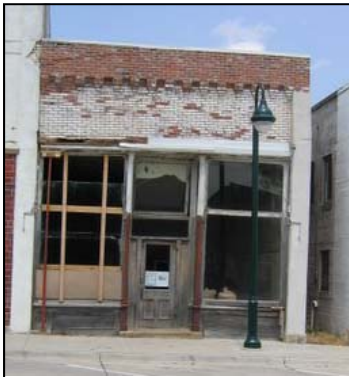
Central City Mainstreet in Iowa received a Hart Family Fund grant to help pay for a structural assessment of the downtown Gambles Building. Hart Family Funds are available to applicants in towns with a population of less than 5,000.
