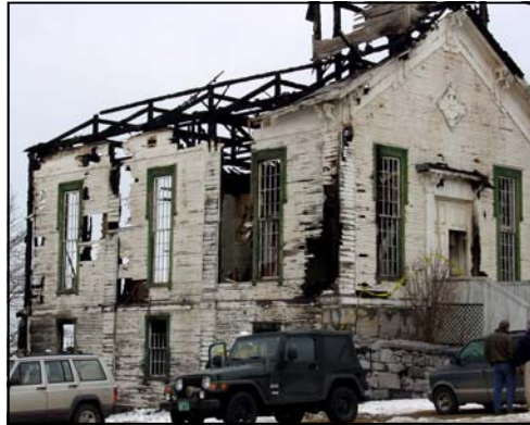
The Grange, days after a devastating fire.
