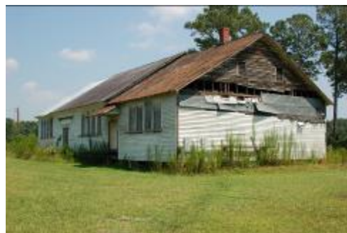
AFTER RESTORATION, HAMILTON SCHOOL WILL SERVE AS A CANOE AND KAYAK OUTPOST AND INTERPRETIVE CENTER FOR THE ROANOKE RIVER PADDLE TRAIL SYSTEM.
