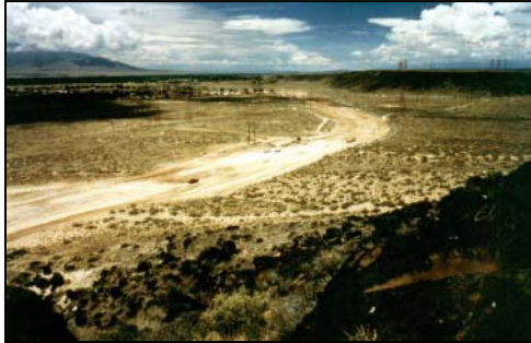
Construction of Unser Boulevard as it winds along the edge of Petroglyph National Monument, NM. [NTHP]
