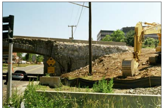
Construction activities have already damaged the stone fascia of the historic Main Avenue Bridge. Connecticut DOT has agreed to stop bridge demolition activities until after the court hearing on Sept. 27.
