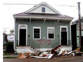
Home in New Orleans damaged as a result of Hurricane Katrina. [NTHP]
