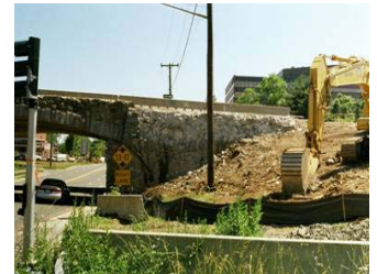
Construction activities had already damaged the historic Main Avenue Bridge before Connecticut DOT agreed to cancel the construction contract and reevaluate the project. [NTHP]
