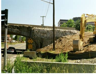
Construction activities had already damaged the historic Main Avenue Bridge before Connecticut DOT agreed to cancel the construction contract and reevaluate the project. [NTHP]
